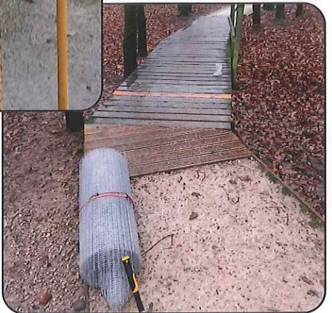
Right: Path repairs were actioned on the wooden walkways at the Millennium Green
